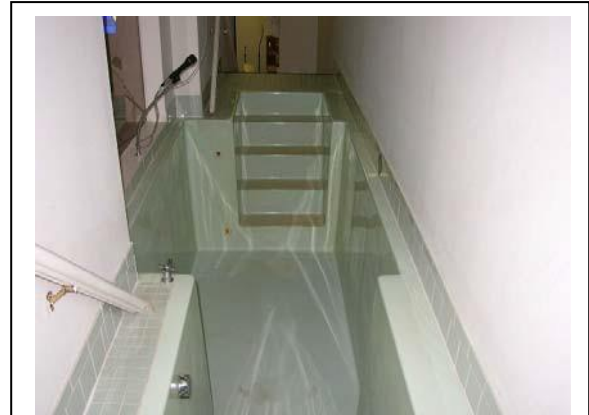
This photo illustrates a corded microphone installed in the baptistry. The risk of electrocution is present for anyone in the baptistry who could contact the microphone. The microphone in this photo should be relocated and suspended from the ceiling or replaced with a cordless microphone.
